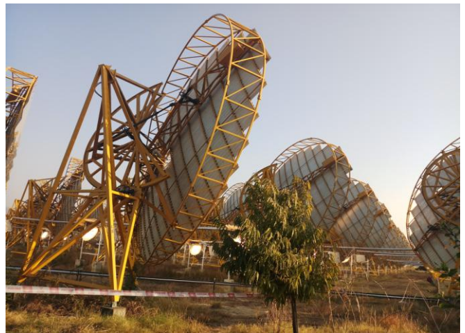
Figure 1: “India One” Solar Thermal Power Plant, Abu Road, Rajasthan
